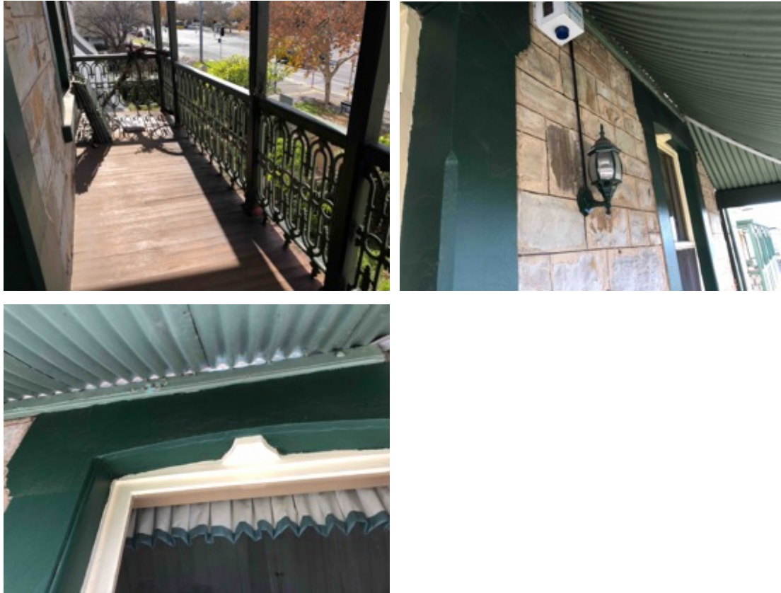
Figure 38 Dilapidation Inspection: Balcony Source: Flightpath Architects, July 2018.
