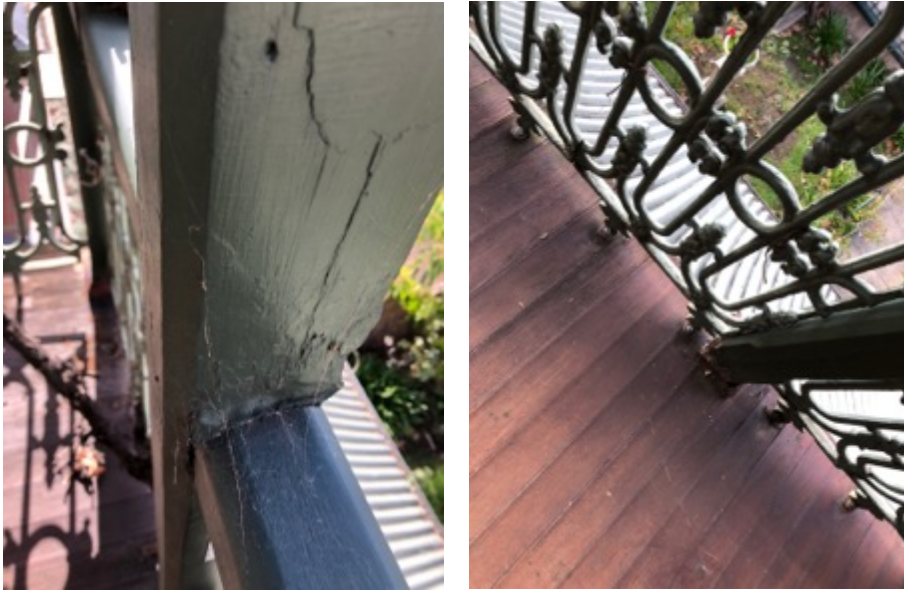
Figure 26 Existing balcony in poor state of repair, Flightpath Architects, 2017 Source: Flightpath Architects, 2017
