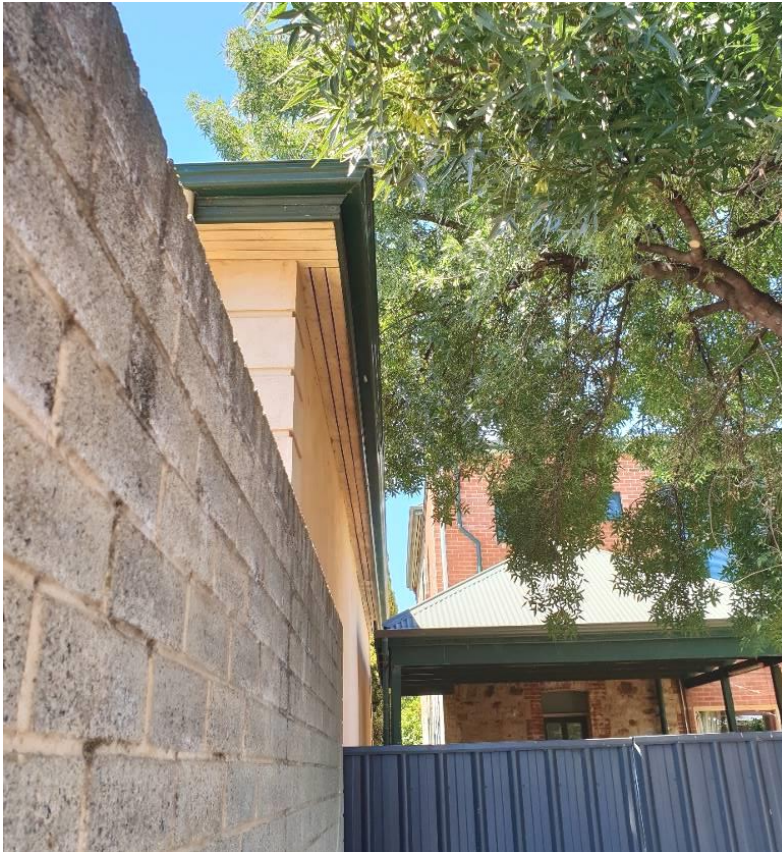
Figure 3 – Gutter at 95 Jeffcott Street extending over northern boundary of subject site
