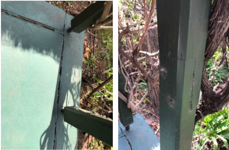
Figure 41 Ground Floor Verandah Posts and cracked verandah slab Source: Flightpath Architects, July 2018.
