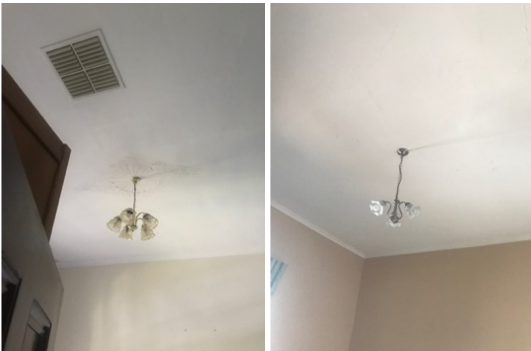
Figure 18 Non-original ceiling, cornice, light fitting and air conditioning Source: Alexander Brown Architects, 2017.
