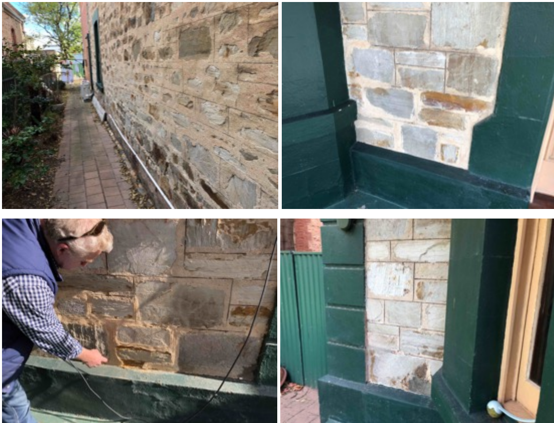
Figure 42 Repointing extent Ground Floor side and front walls Source: Flightpath Architects, July 2018..
